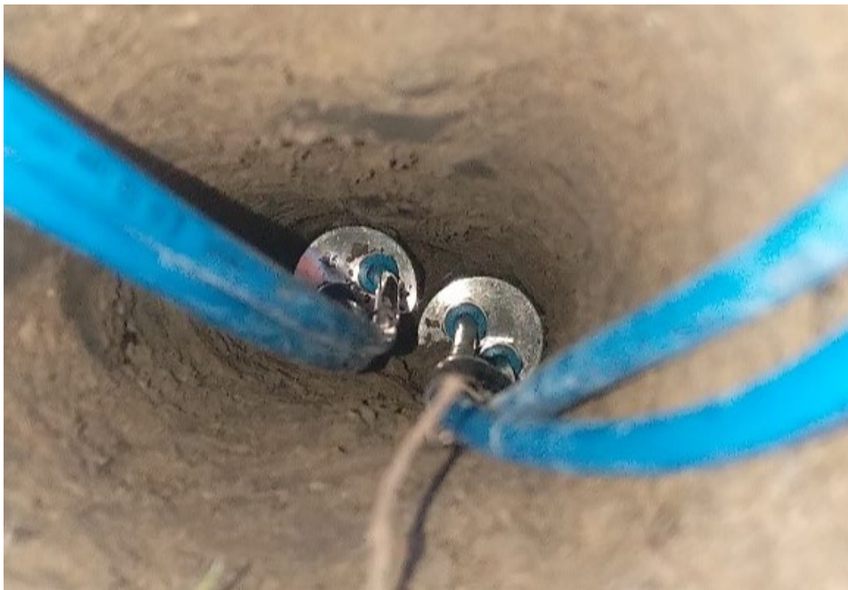
Figure 2. Tests of two cylindric radon probes prototype in a 2x10 cm hole at a depth of 0.9m.
