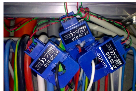
Figure 2. Hall sensors on Building D Light.
